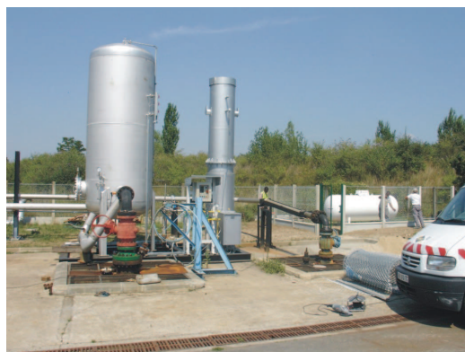
Fig. 4.5.5 Solution gas degassing/abatement facility (source: GPC IP, 2002).
