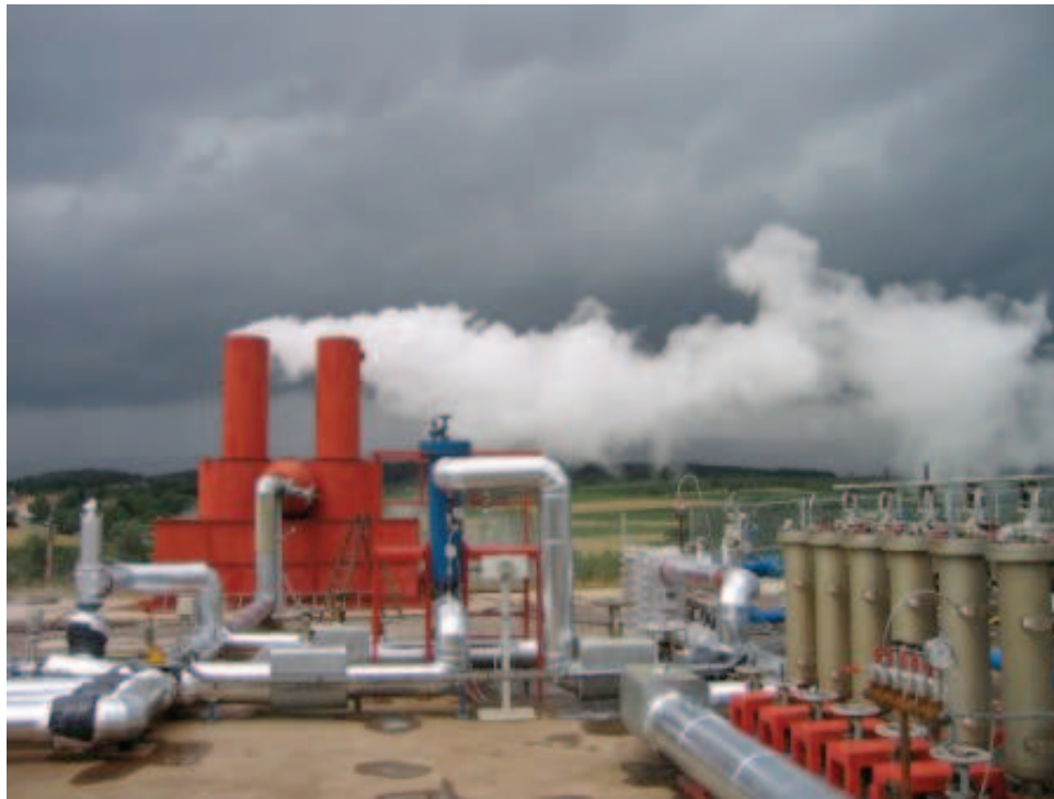
Fig. 4.7.3 – Soutz EGS project. Circulation test facility (source: ENGINE, 2006).
